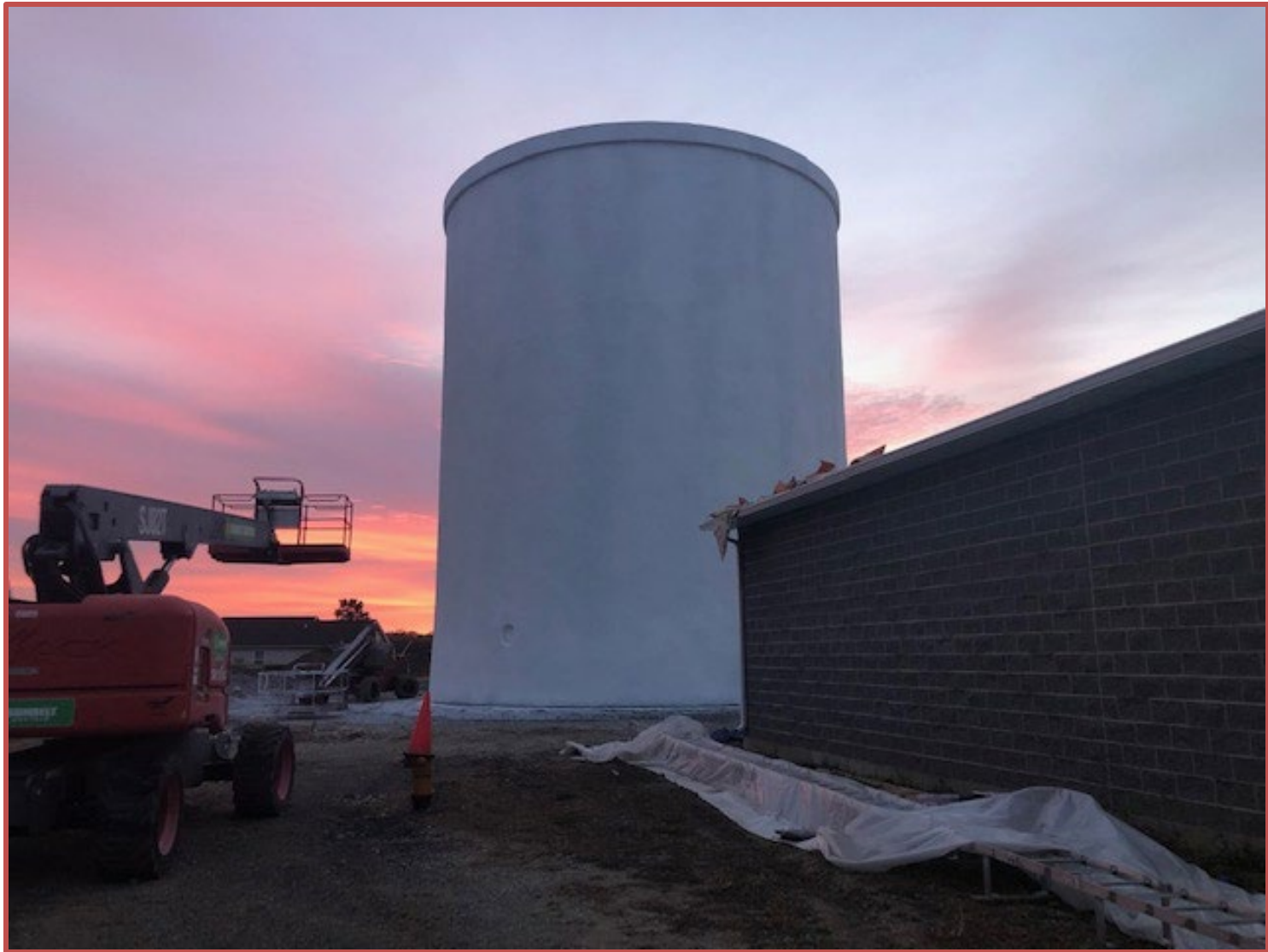
Image 6: Armory Road Ground Storage Tank and Booster Station
